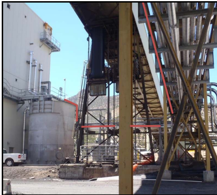
Figure 5 – Dewatering to Pug Mill Pipeline
