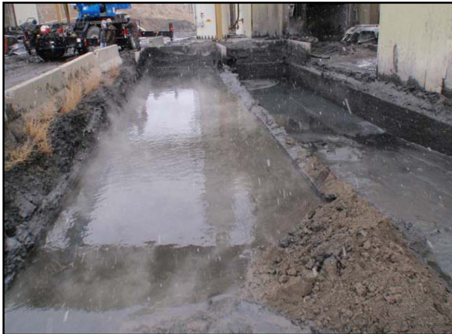
Figure 7 – Pug Mill Wash Down Settlement Basins
