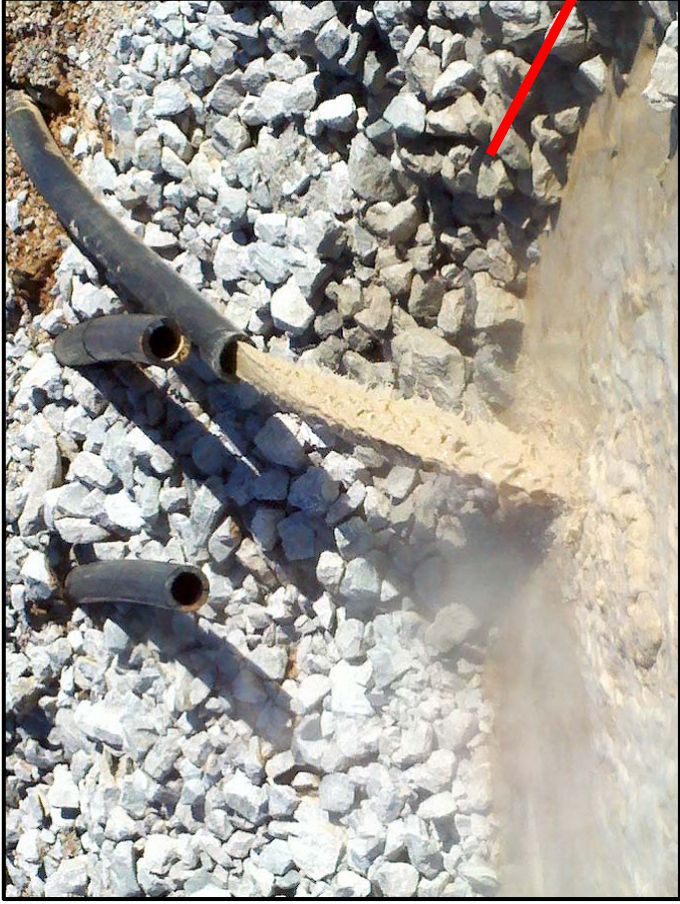
Incoming Gypsum Slurry (during initial wet operation)
