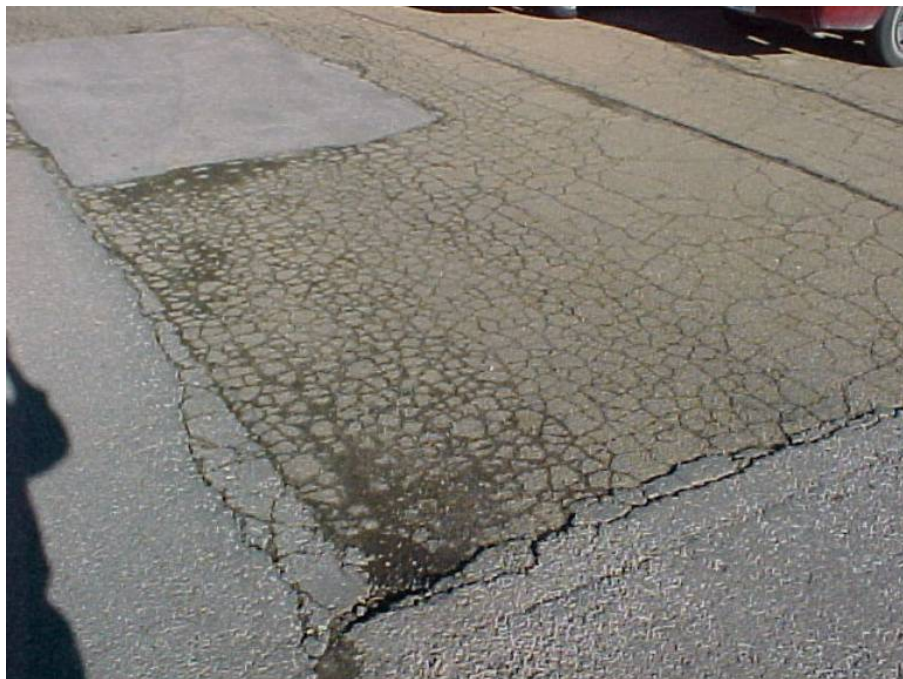
Figure 4. Alligator cracking with large patches
