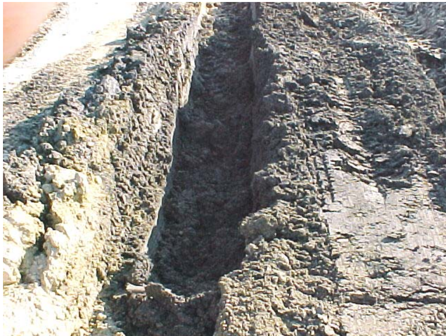
Figure 7. Severe rutting due to unstable subgrade
