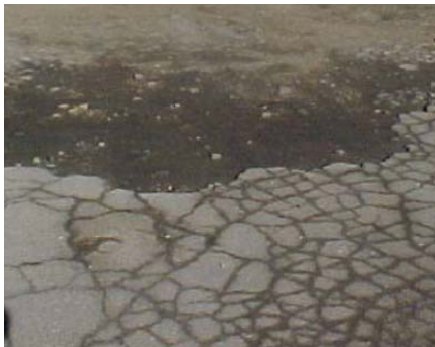
Figure 2. Existing asphalt pavement showing pothole and fatigue cracking
