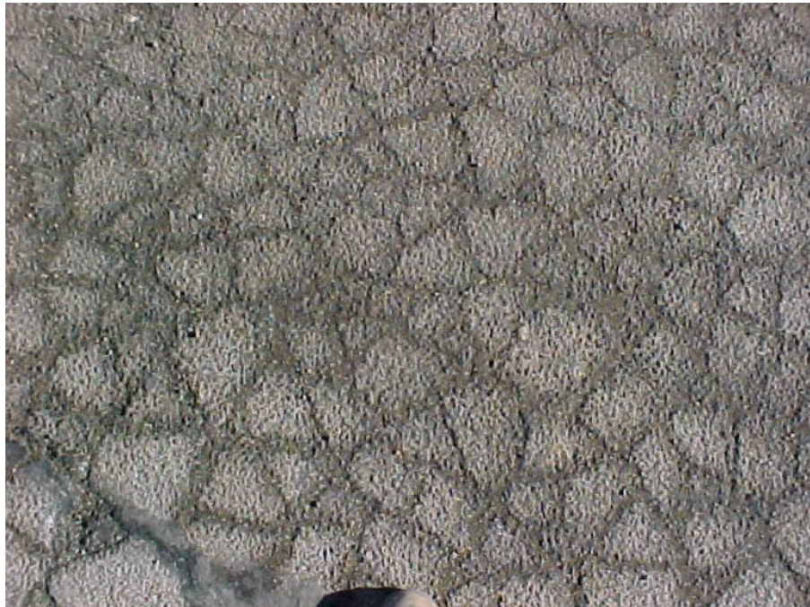
Figure 3. Severe alligator cracking
