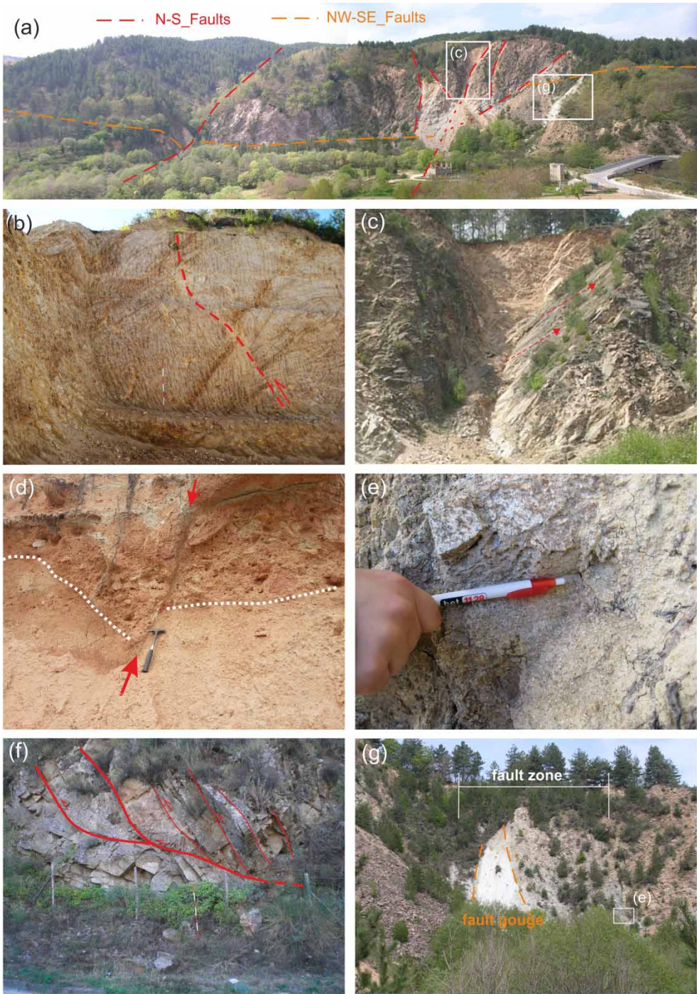
Figure 6. Examples of faults surveyed in the study area at the macro- and meso-scale: (a) panoramic view of the right slope of the Arvo river and some faults related to the main fault systems; (b) N-S transpressive faults; (c) N-S right-lateral transpressive faults; (d) last kinematics on the N-S fault plane in the Pleistocene conglomerates; (e) left-lateral striae on the NW-SE fault plane; (f) ancient overthrust; (g) NW-SE fault zone with associated thick fault gouge.
