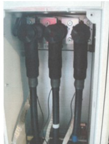
Fig. 3. HV terminal and connectors connected to 6.6 kV breaker system.
