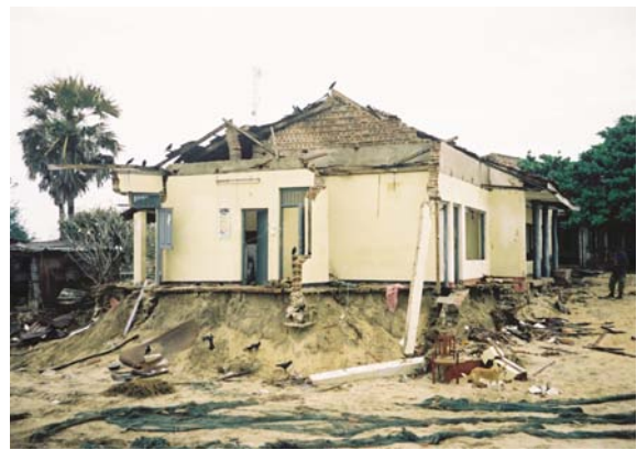
Fig. 7. The soil erosional action of the tsunami caused the sea-facing side of the non-RC building to collapse ( \sim 120 m from beach, near Karativu, east Sri Lanka).
