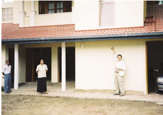
Fig. 5. Two-storey RC house that resisted very well the tsunami attack at distance of \sim 80 m from the shoreline of Paralyia, southwest Sri Lanka. Only little damage was caused in doors and windows. Water mark was left on wall.
