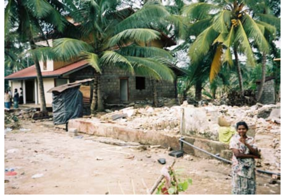
Fig. 6. Non-RC brick-work house completely demolished by the tsunami in Paralyia, southwest Sri Lanka. In the left-hand side the RC house (Fig. 5) makes strong contrast.
