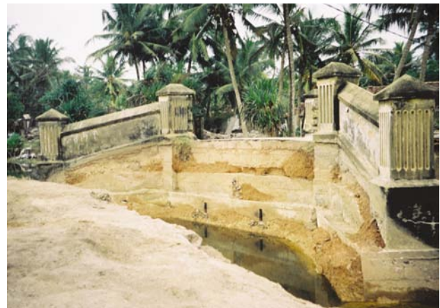
Fig. 10. The soil erosional action along with the force of the hydrodynamic flow of the tsunami caused collapse of one side of bridge (North Kalutara, southwest Sri Lanka).
