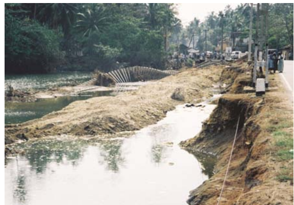
Fig. 8. Complete failure of railway due to lateral spreading and collapse of its embankment caused by the soil erosional action of the tsunami (Abalangoda, southwest Sri Lanka). The tsunami wave moved from the right-hand side to the left-hand side of the picture.
