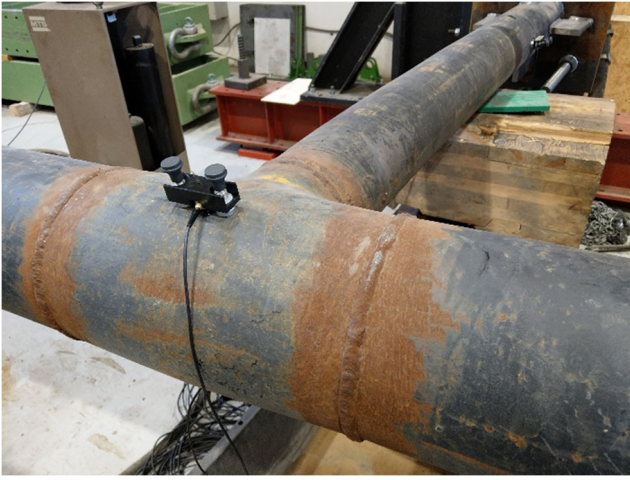
Fig. 16 Acoustic sensor installation on the Tee joint. Typical MAG4M magnetic spring clips used to attach the VS150 sensor on the pipeline
