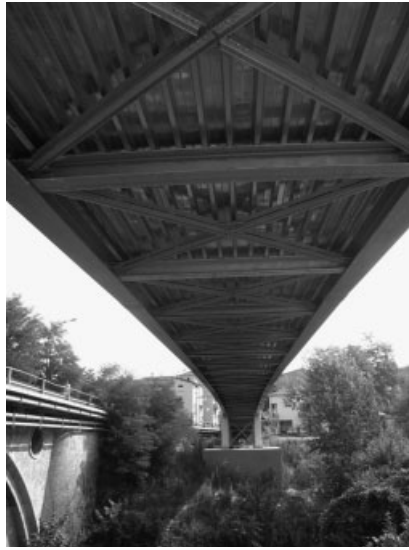
Figure 6. The view of the bridge inferior surface from a position similar to that of the radar device.
