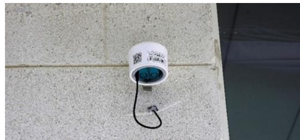
Figure 2. Example of a sensor installation at the University of Pavia
