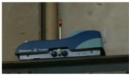
Figure 16. Trolley during operation on a rail of an overhead bridge crane
