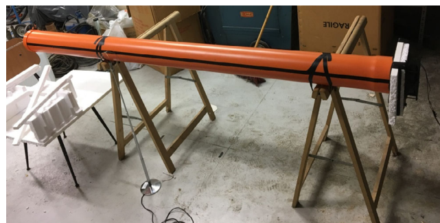
Figure 1. Microventilation system created for the cellar.
