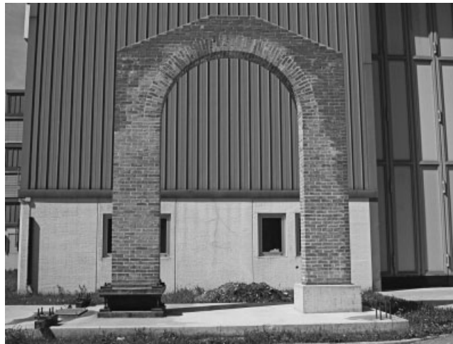
Figure 14. Wet arch due to rain.
