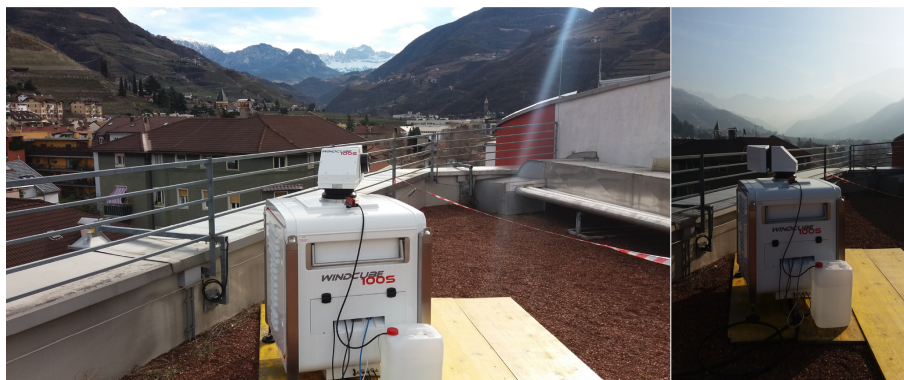
Figure 4. The WINDCUBE 100S Doppler wind lidar from Leosphere (France) installed on a roof at 18 m a.g.l. In the background is the outlet of the Isarco Valley.
