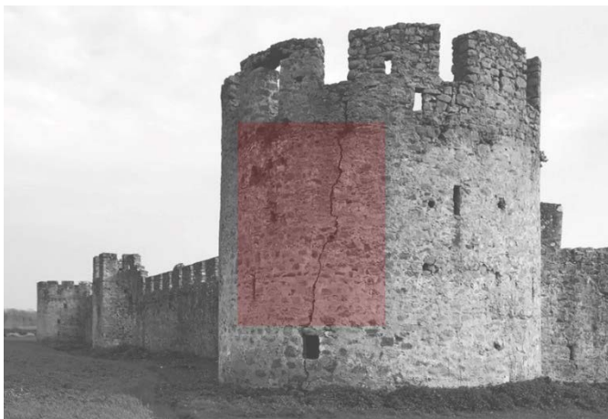
Fig. 2. North tower of the Fortress of Bashtovë. The red portion identifies the analysed area.
