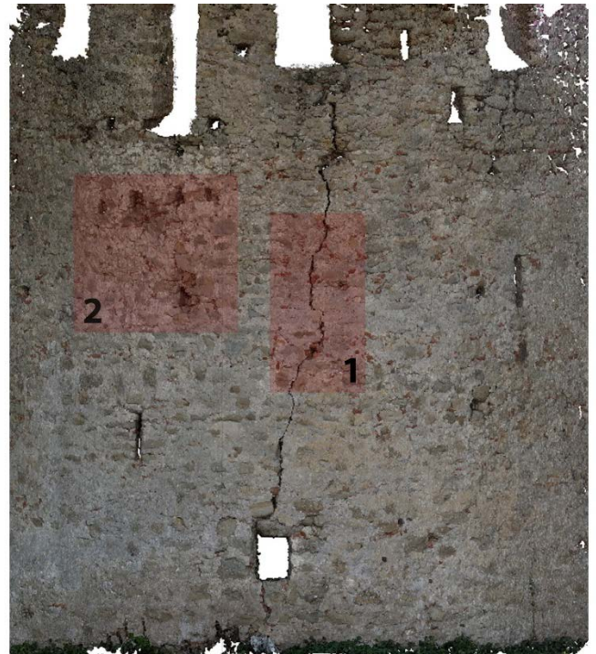
Fig. 3. Point cloud of an extended portion of the north tower (covered area of about 60 m 2 ), with the indication of the two samples (1, 2) used for the application of the methodology.
