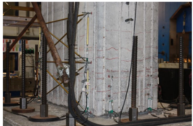
FIGURE 21 Crack pattern at the base of the physical pier after Test HE-70
