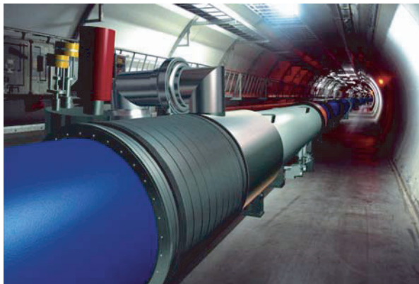
Figure 8. LHC tunnel: cryostat encloses all lattice magnetic elements. Part of a connection box shows at left. The He feed line is hidden behind the cryostat [41].
