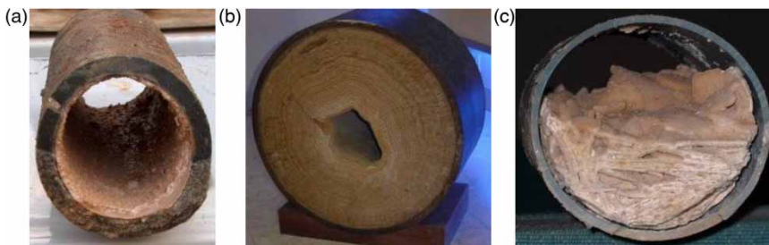
Figure 1 | Pipe cross-section narrowing due to partial blockage features for metallic pipes: (a) and (b) diameter decrease caused by the regular deposit of sediment on the inner walls; for polymeric pipes: (c) accumulation on the lower part of the pipe section of material detached from the walls (Alegre & Covas 2010).
