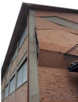
(a) OOP damage of external infill panel (MI.2a).
