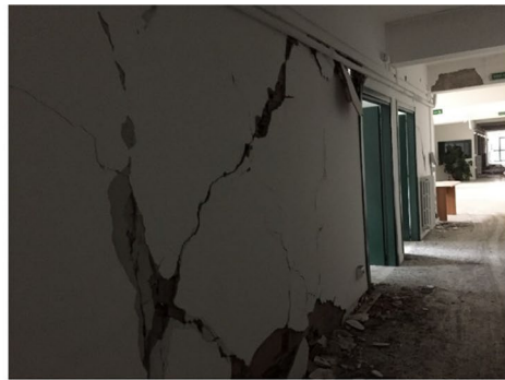
(b) IP damage of internal partition walls.
