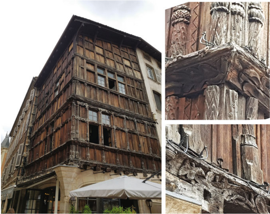
Fig. 3.10 Oldest wooden building in Mâcon (France), dated from the late fifteenth to early sixteenth century—La Maison du Bois, Mâcon, France. Image courtesy of Wim Willems—FirmoLin
