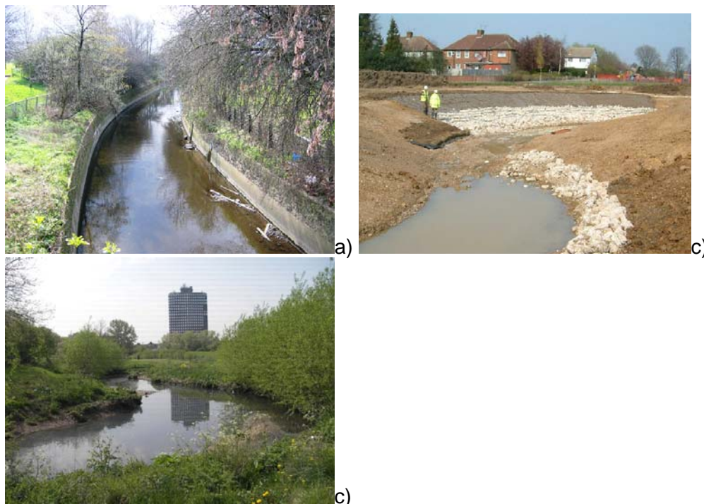
Figure 10.4 Images from hard bank removal on the River Trent in London. a) concrete-lined channel before restoration, b) construction of riverbed and banks after concrete removal, c) natural vegetation and bank features.
