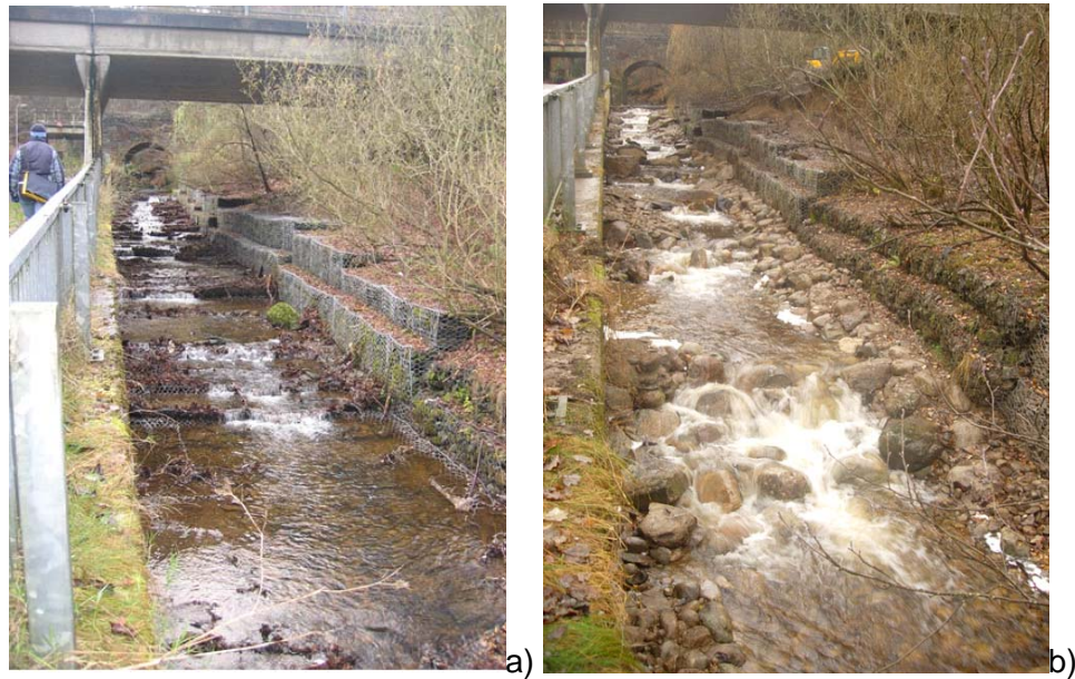
Figure 10.5 Case study of boulder placement restoration. a) before restoration activities, b) after boulder placement (from RRC).
