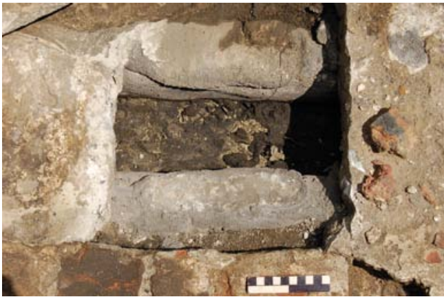
FIG. 105 Detail of a channel with muddy silt after removal of the cover.
