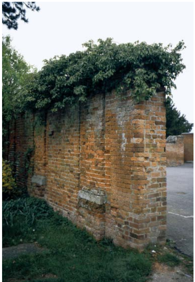
FIG. 21 Careful analysis of the form and fabric of surviving walls can lead to the identification of parts of lost structures such as this fragment of an 18th-century orangery now in the grounds of Shaw House School, Newbury in England.
