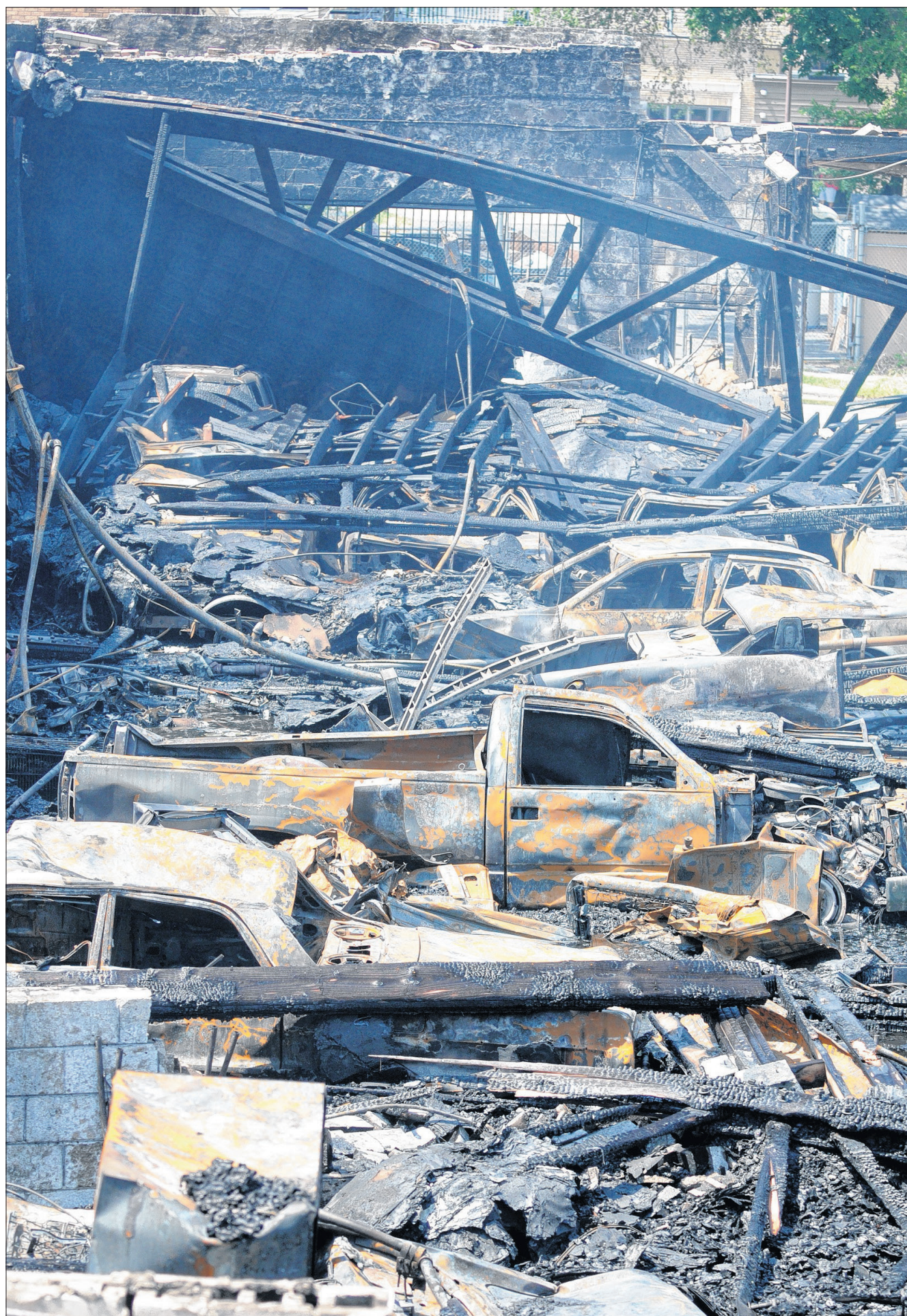
A total of 25 fire-damaged cars sit inside the burned-out remains of the building at 609 E. Court St. in Kankakee after a devastating early morning fire Thursday.
