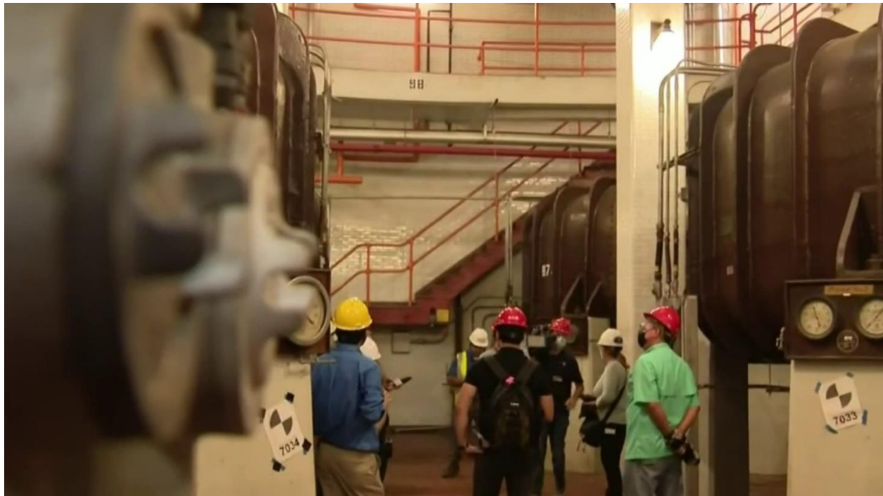
Conner Creek Pump Station
