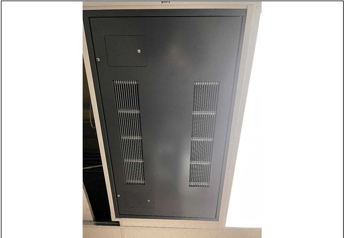
Photograph: 9 Main ceiling air vent.
