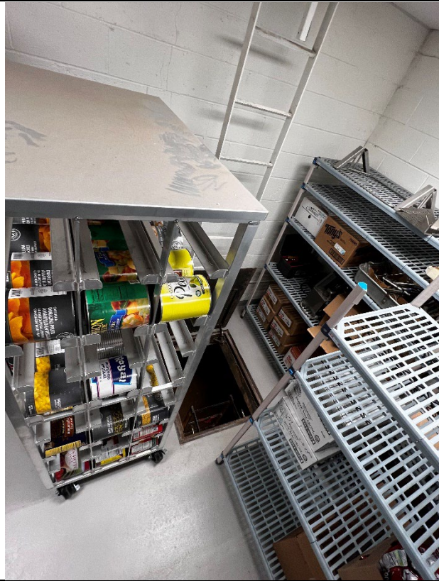
Photograph: 15 View of crawl space access opened, taken from middle of storage room.
