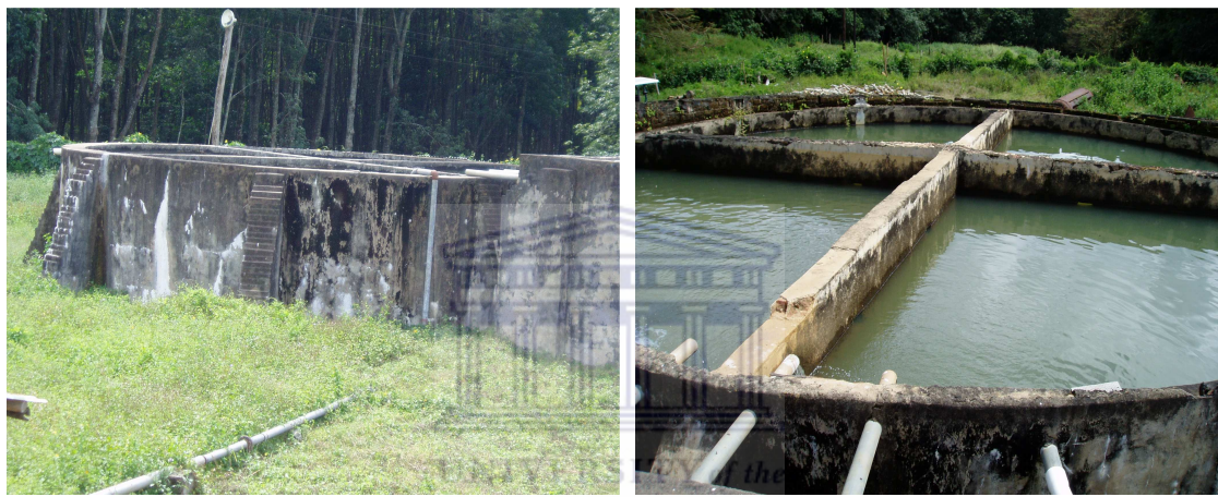
Figure 21: 5.7 Water storage tank at Vizara Rubber Plantation Factory (water use)
