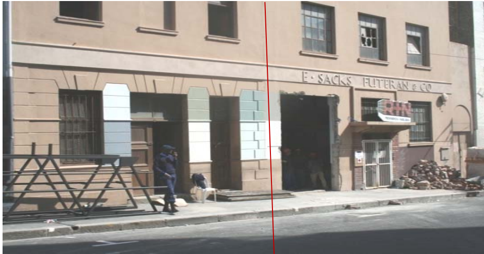
Figure 56 Two warehouse buildings: no.14 & 16 Harrington Street - Part of E. Sacks Futeran & Co. during renovations. District Six Museum archive.
