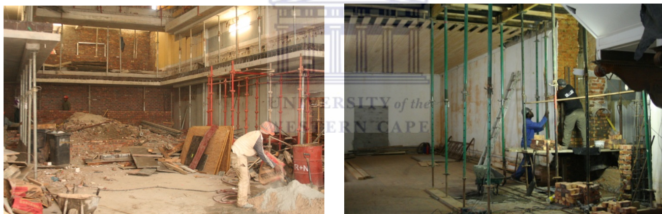
Figure 60 Creating new theatre spaces and installing new ceilings and openings between the two Buitenkant Street warehouse buildings. District Six Museum archive.
