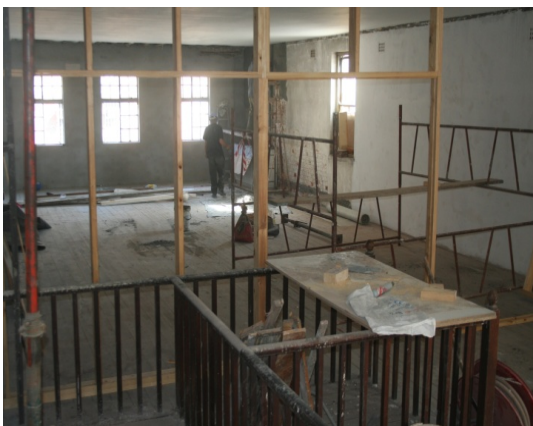
Figure 63 Constructing interior frames for new wall of archival storeroom in c1903 warehouse building. District Six Museum archive.
