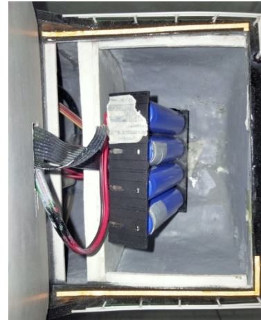
Power Battery Area Buritan
