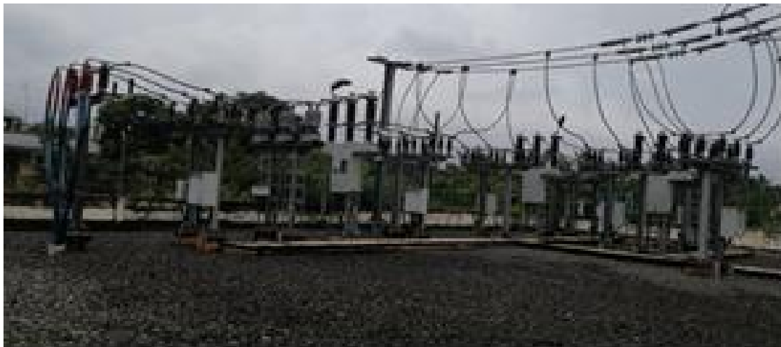
Figure 1: A primary substation
