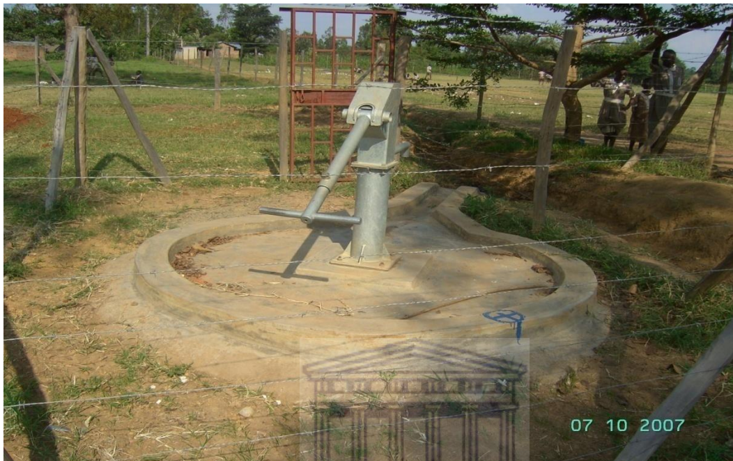
Figure 5.4 Photograph of a CDF Water Project at Burumba Primary School
