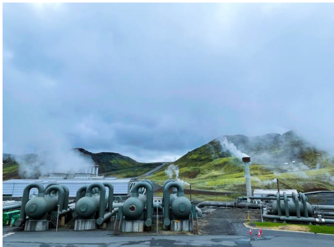
View at the Hellisheiði plant
