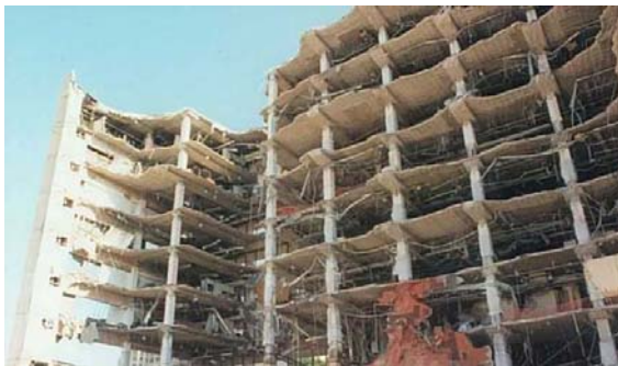
Figure 2.2.a. Murrah Building showing the damage after the debris was removed
