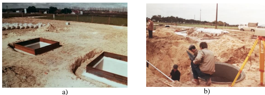
Figure 5. Installation of drainage lysimeters (a, left) before insulation, visible the thin upper wall and, in distance, the bags containing the soil extracted by layers for refilling and (b, right) installation of the pipes bringing the drained water to the wells where water flow would be recorded (1984, Coruche, Portugal).
