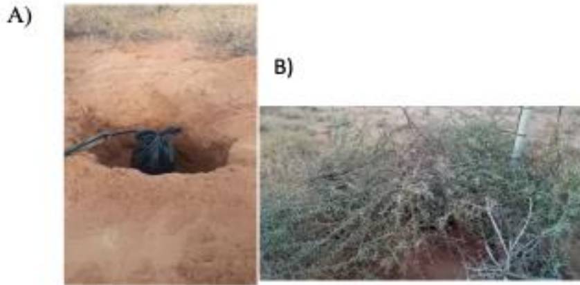
Figure 3.1. Photos showing the installation of the Seismometer in the BUR station where panel A shows the digging for the installation of the seismometer and panel B shows the backfilling and the covering of the hole.
