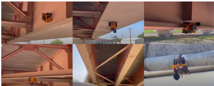
FIGURE 5.31: Robot deployment on a bridge on Highway-80 located in Lovelock city, NV, USA. The robot traverses upside down on the main I-shape beam; the Robot passes an edge of the I-shape beam; the Robot moves upside down on a T-shape member, and the robot travels stably on a bridge water draining tube.
