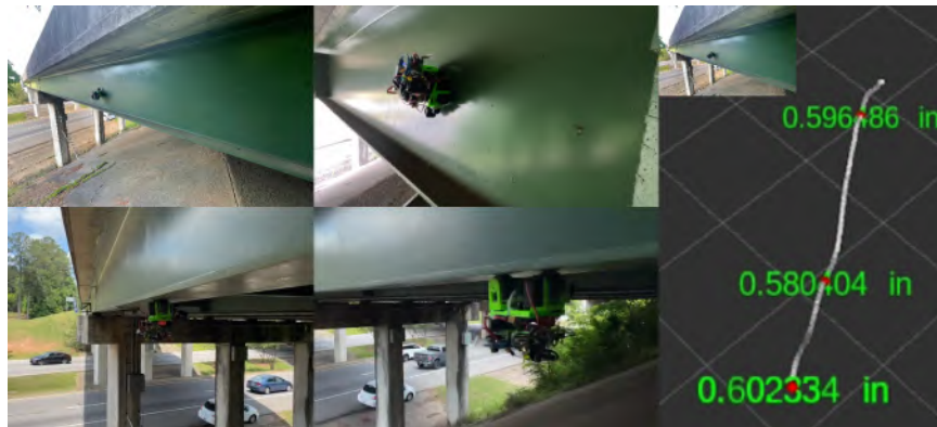
FIGURE 5.33: Robot deployment and data collection on a bridge on Highway I-75 in Georgia, USA. Robot positions and steel thickness data are synchronized in real-time. The robot path represents in white color. Steel thickness measuring positions are red dots. Thickness data (numbers in green color) is shown in inch units.
