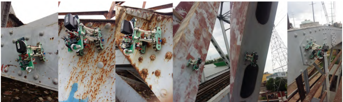
FIGURE 2.25: Adhesive and climbing test on a rusty paint-coated steel bridge: flat structure with bolts/nuts.
