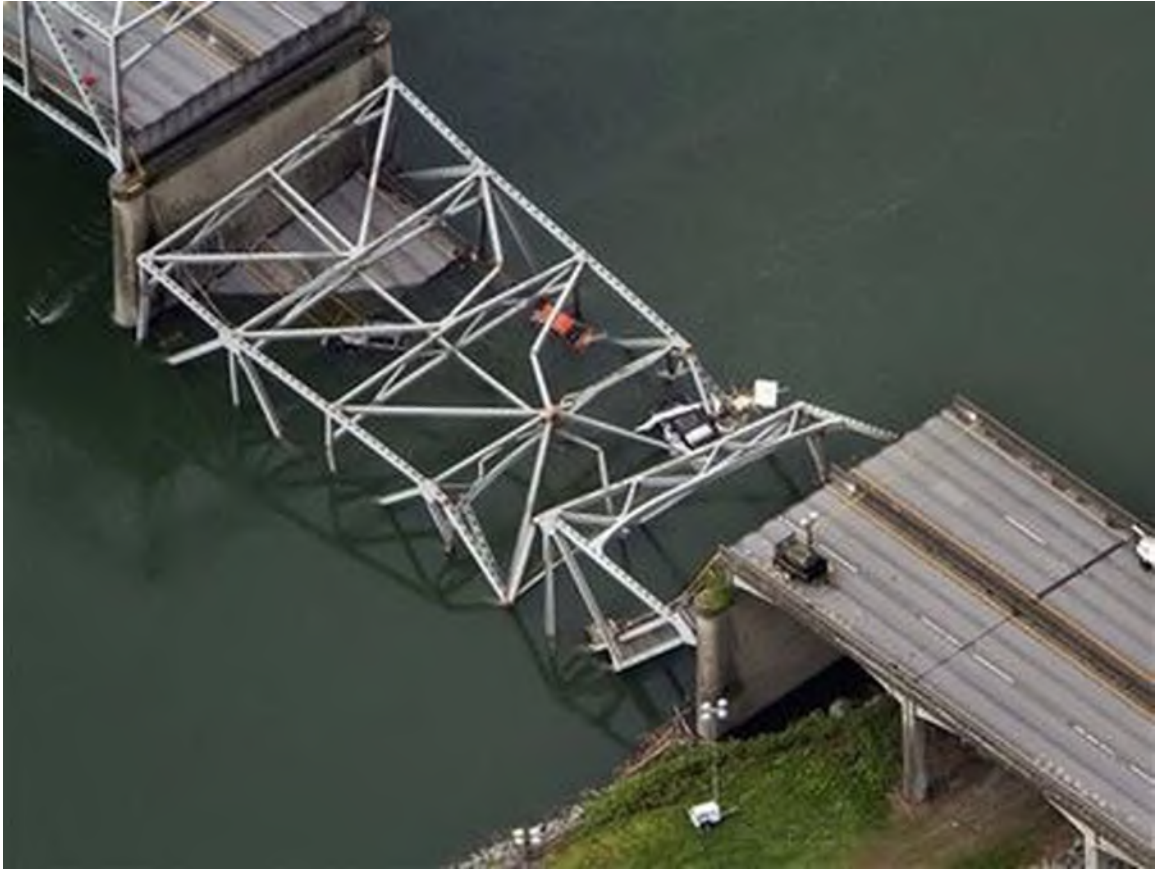
FIGURE 1.2: A collapsed section of the Interstate 5 bridge over the Skagit River is seen in an aerial view Friday, May 24, 2013, in Mt. Vernon, Wash. (Source: Google images)
