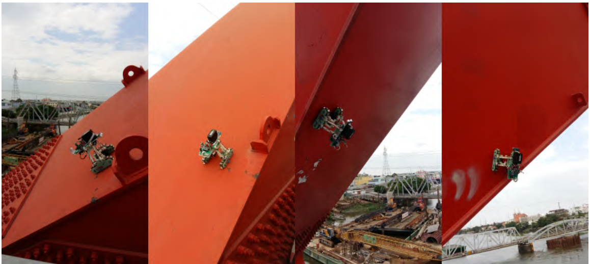
FIGURE 2.24: Adhesive and climbing test on a thick paint-coated steel bridge: a flat surface.
