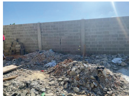
Figure 1: Waste produced by the demolition of the slab and column structural elements.
