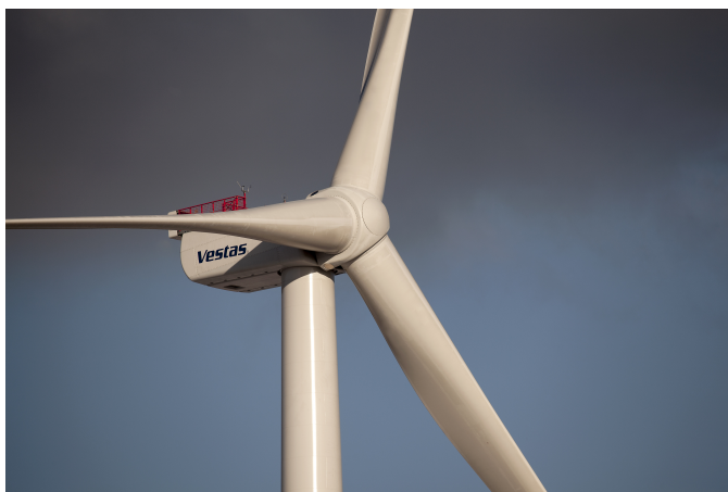
(a) Vestas V164-8.0MW installed
