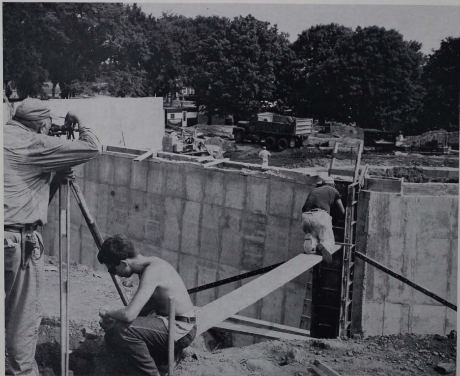
Surveying engineer takes sight of dining hall foundation. Tennis courts can be seen in the background, left.
