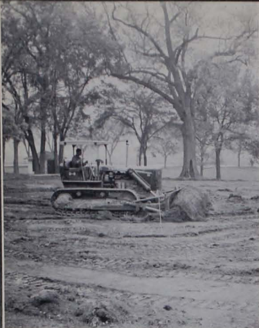
Bulldozer pushing off top soil for construction of the new dining hall.
