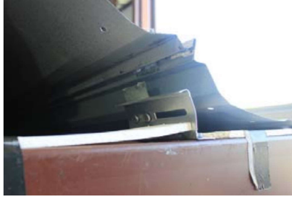
Figure 25: Clip rupture and breakage at the clip-seam connection due to panel deflection and deformation (Habte et al., 2015).
