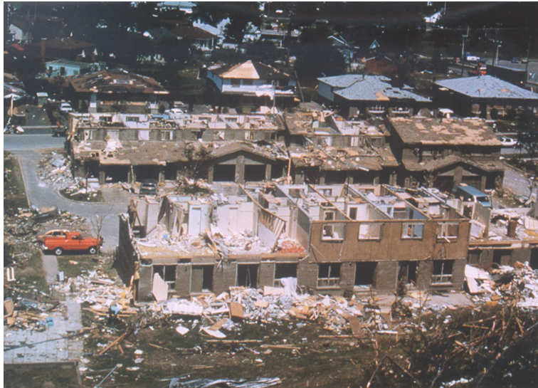
Figure 1: Photograph of compromised houses from damage survey from the Barrie Tornado in 1985.
