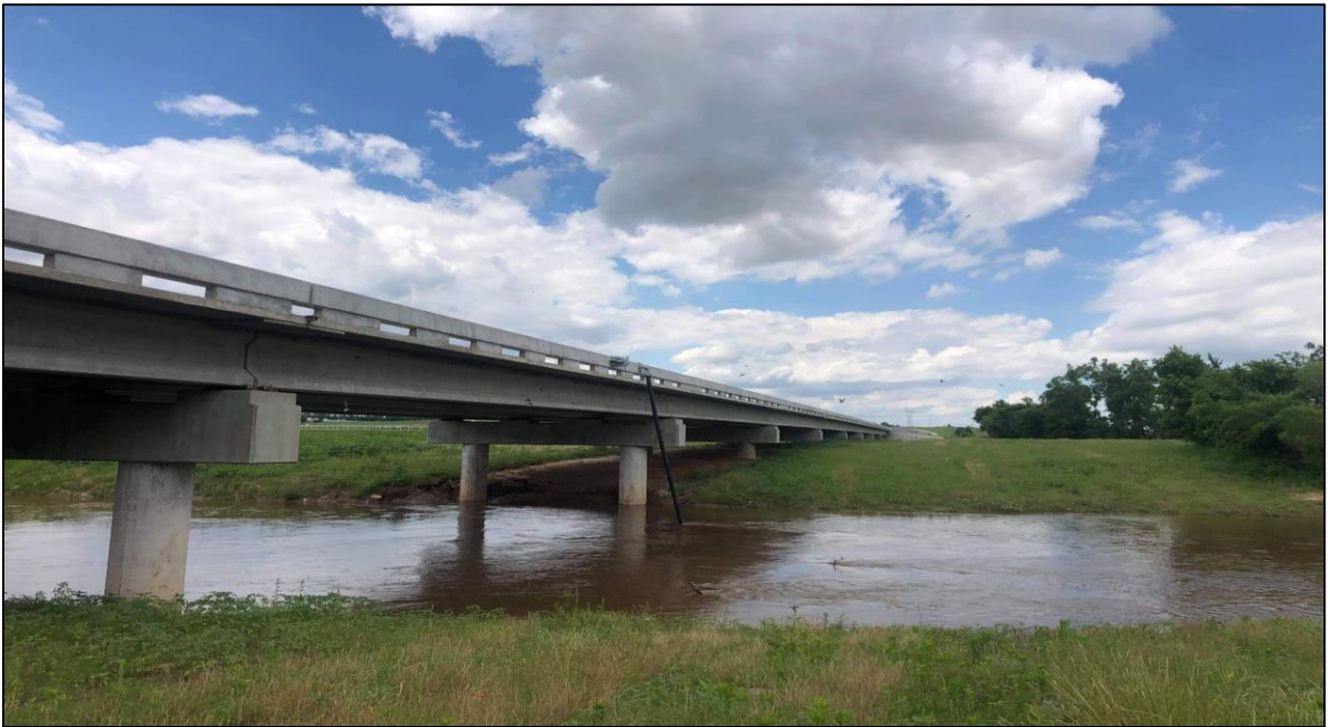
Figure 3.10: Photograph of the SH 4 Bridge over N. Canadian R., Canadian Co., OK.
