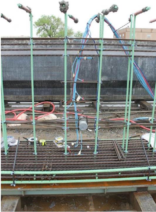
Figure 3.17: Instrumentation at midspan, Mark 27, Span 9. Four #7 reinforcing bars are placed in the corners of the bottom flange.
