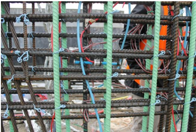
Figure 3.16: Vibrating Wire Gauge (blue) is located in the foreground at approximately C.G.S.
