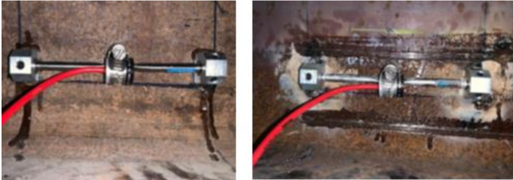
Figure 3.3: Geokon model 4000 VWSGs welded and glued to the steel beam of the prototype bridge
