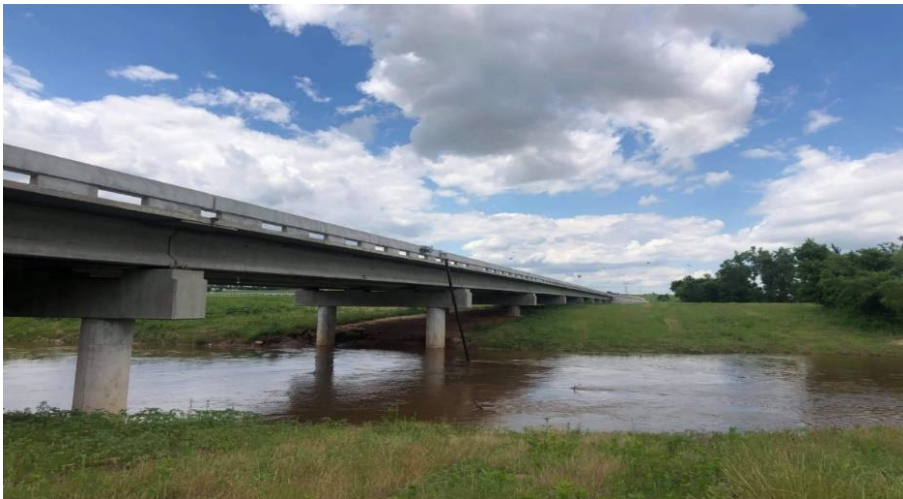
Figure 4.1: Photograph of the SH 4 Bridge over N. Canadian R., Canadian Co., OK.
