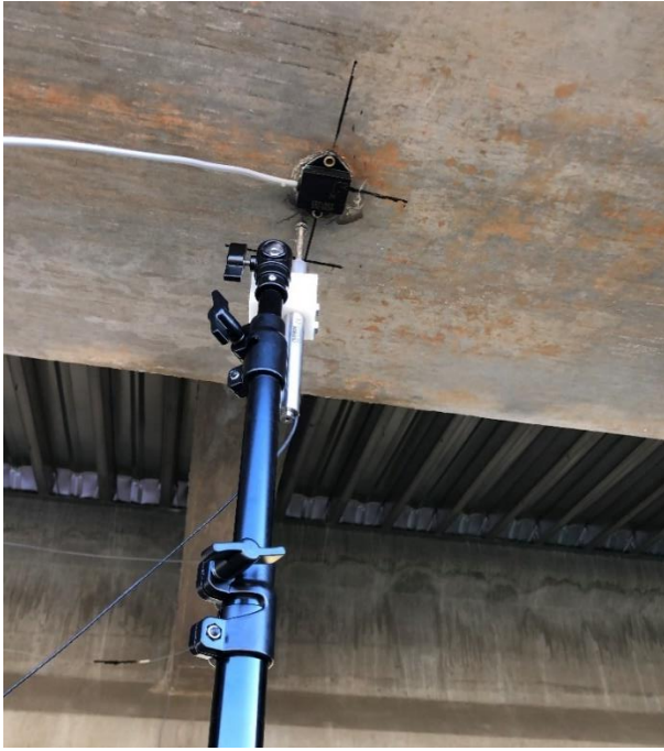
Figure 6.4: Instruments at midspan for SH 4 load test. Viewed are an LVDT and accelerometer.
