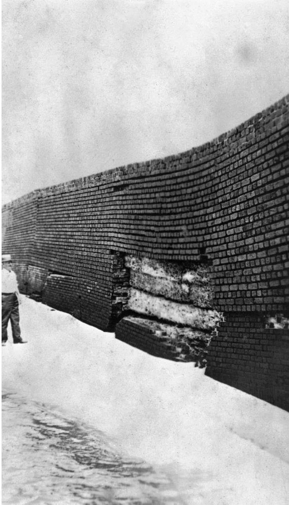
Figure 18: Tidal damage to a wall at Fort Clinch, circa 1930. (State Archives of Florida)
