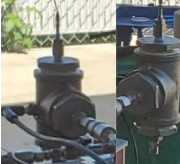
Figure 9 : Pictures of Combustion Chamber
