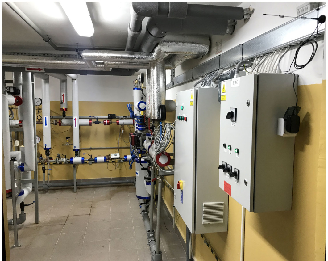
Figure 2. Control room in the building where tests were performed. On the right-hand side there are two control cabinets. The smaller one is a heat substation switchgear. The larger cabinet contains Honeywell Excel Web Ethernet-based programmable building automation controller, Weintek cMT-SVR-100 data logger, Ethernet switch, and an edge router for wireless sensors connected to an antenna visible in the upper right corner. In the background is the hydraulic installation: vertical pipes are for domestic hot water, horizontal pipes are for primary side district heating. A Kamstrup Multical 603 energy meter is visible straight ahead. On the right-hand side, behind the cabinets, there is a cylindrical strainer for secondary side central heating return water. Above it, there are two variable speed drive pumps.
