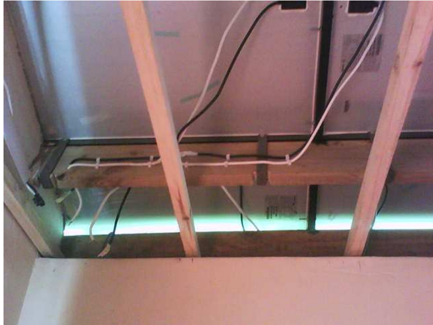
Figure B.9 BIPV back of module view before ceiling installation.
