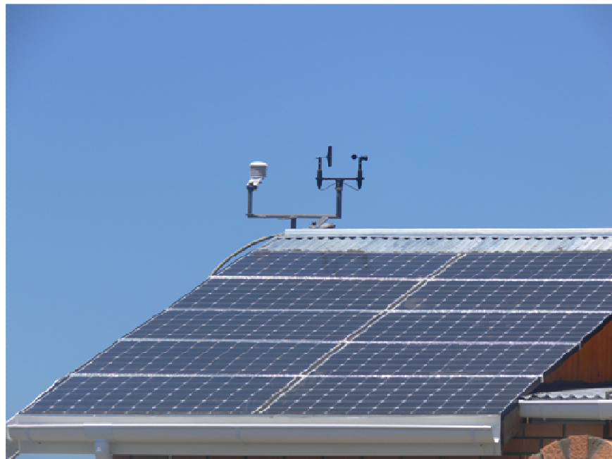
Figure B.10 The eastern PV array and weather station
