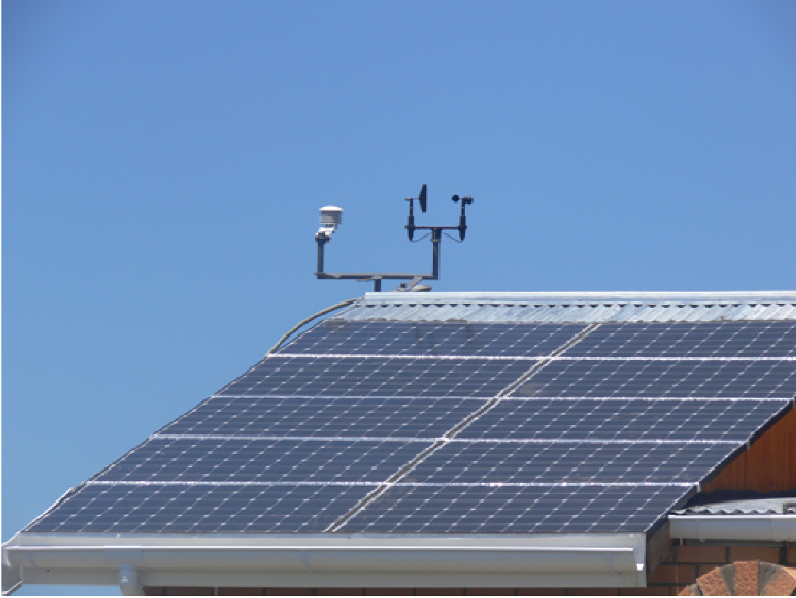
Figure 6. 2 BIPV modules and outdoor weather sensors.
