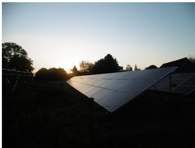
Figure 10-5: Solar PV array at Canon Frome Court cohousing
