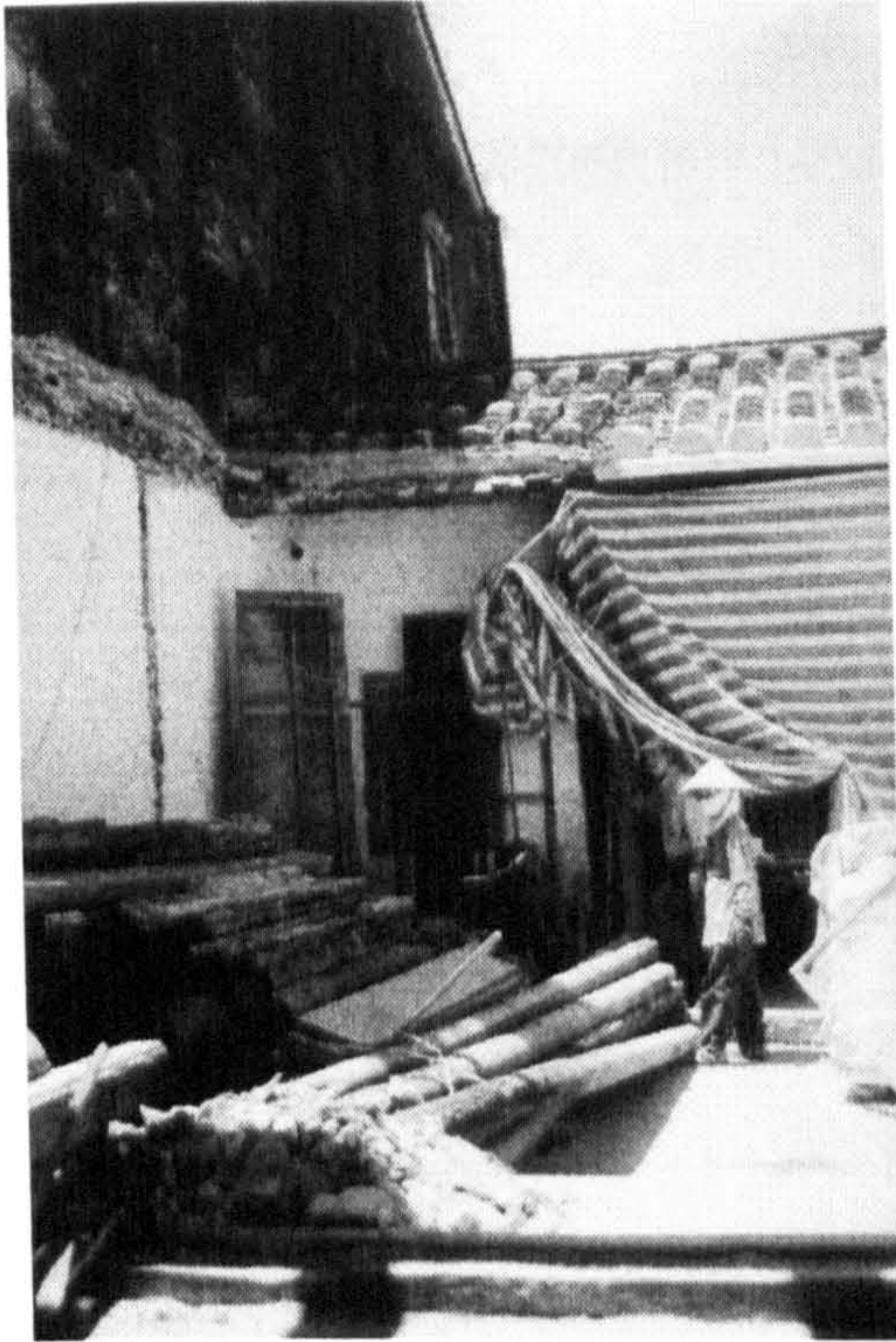
Figure 4.17: Restoration of No. 104 Nguyen Thai Hoc. The timbers were left unprotected and stacked without enough care.
