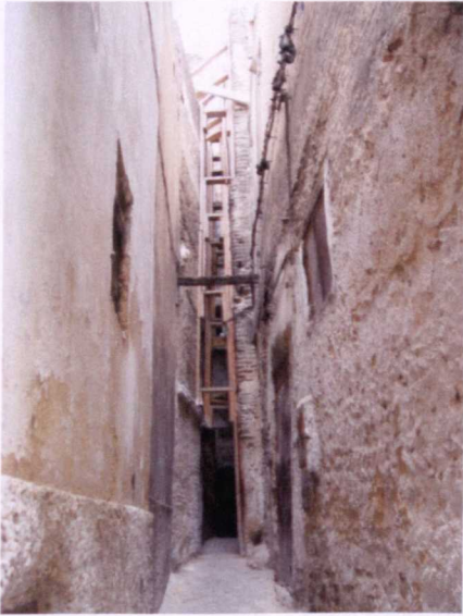
Figure 5-13- A Very Narrow Street in Talaa Saghira, Emergency Interventions to Prevent the Walls from Collapsing Can Be Seen (Picture Taken By the Author, November 2006)
