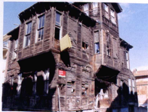
Figure 5-73- Another Deteriorated Building Resided By 6 Families (Photo Taken By the Author in September 2007)
