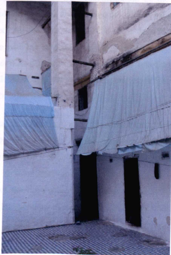
Figure 5-26- A View from another Shared Courtyard House. This House Is Shared Between 7 Families. In This Building, Permanent Walls Are Introduced to Provide Privacy. Guerniz (Picture Taken by the Author, November 2006)
