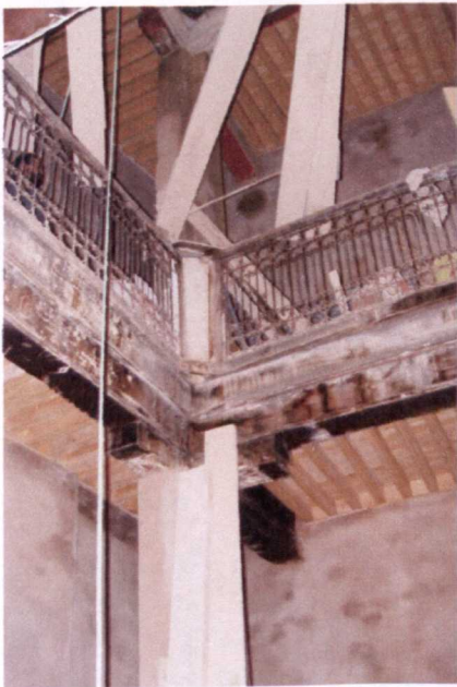
Figure 5-19- A House in Talaa Saghira Which Was Under Restoration Using the Loan from ADER-Fez (Picture Taken By the Author, November 2006)
