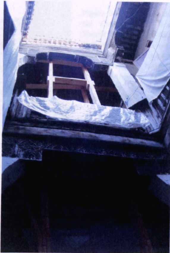
Figure 5-23- View from Inside a Courtyard House Shared By 4 Families. Emergensi Interventions to Prevent form the Collapse of the Building Can Be Observed in the Courtyard As Well As Inside the Rooms. Guerniz (Picture Taken by the Author, November 2006)
