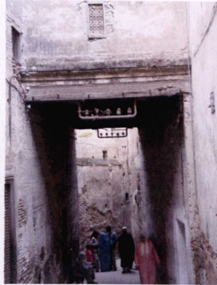
Figure 5-14- A Street in Douh Which Is Covered By a Sbat (Picture Taken By the Author, November 2006)
