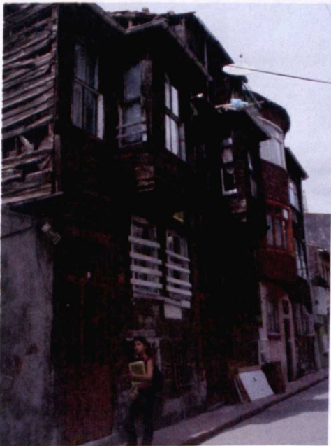
Figure 5-72- This Building Is In Very Poor Condition, But the Owner Has Only Afforded a New Door to Increase Safety (Photo Taken By the Author in September 2007)
