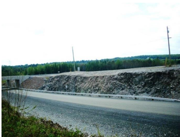
Figure 6. Large outcrop along the Plymouth Road as part of the expansion to Route 95.
