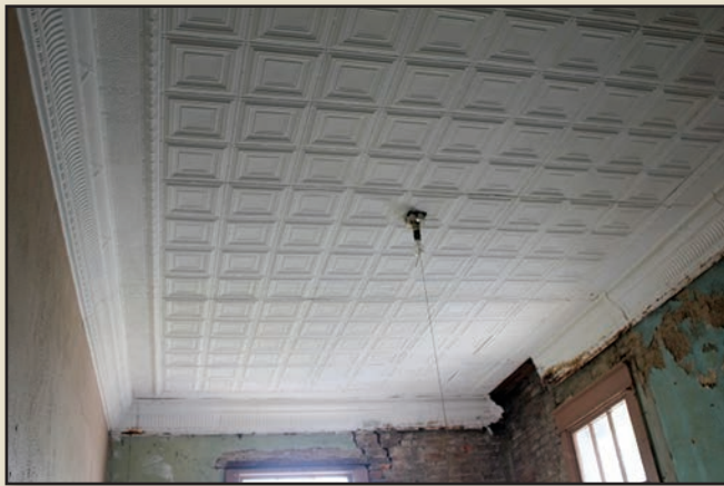
Detail of the pressed tin ceiling in the President's Office of the Red Boiling Springs Bank.
