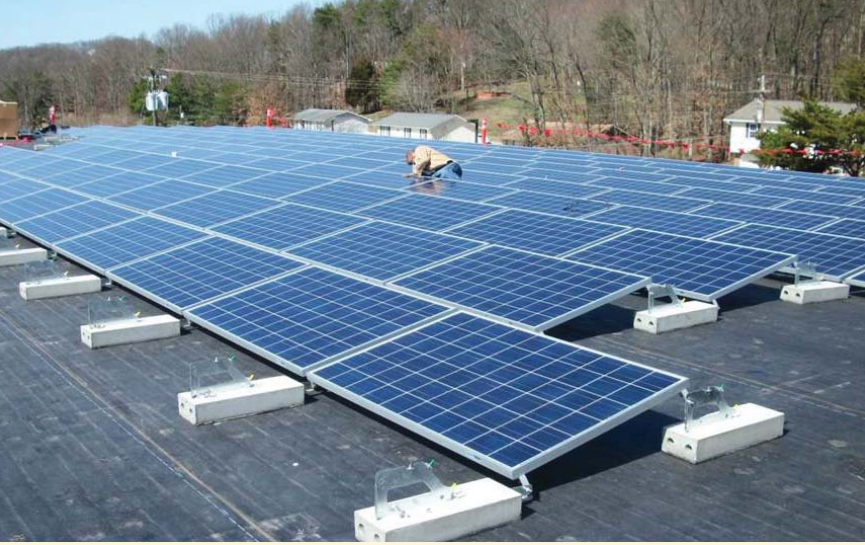
Hawkins County School Solar Project
