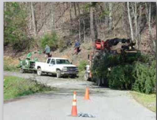
Fuel removed in the Norris Shores Community of Union County makes this community safer from wildfires.
